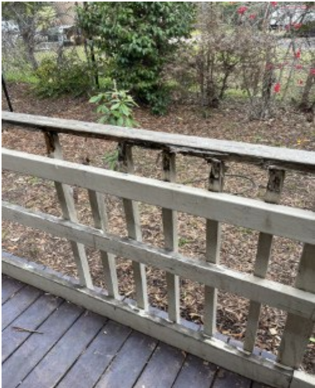
Rotted handrail outside Bldg. 2
