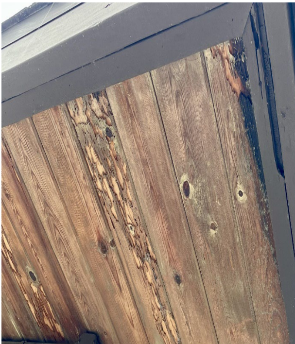
Termite damage and wood rot (Bldg. 1)
