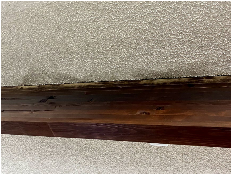
More evidence of water intrusion and possible mold in Bldg.2
